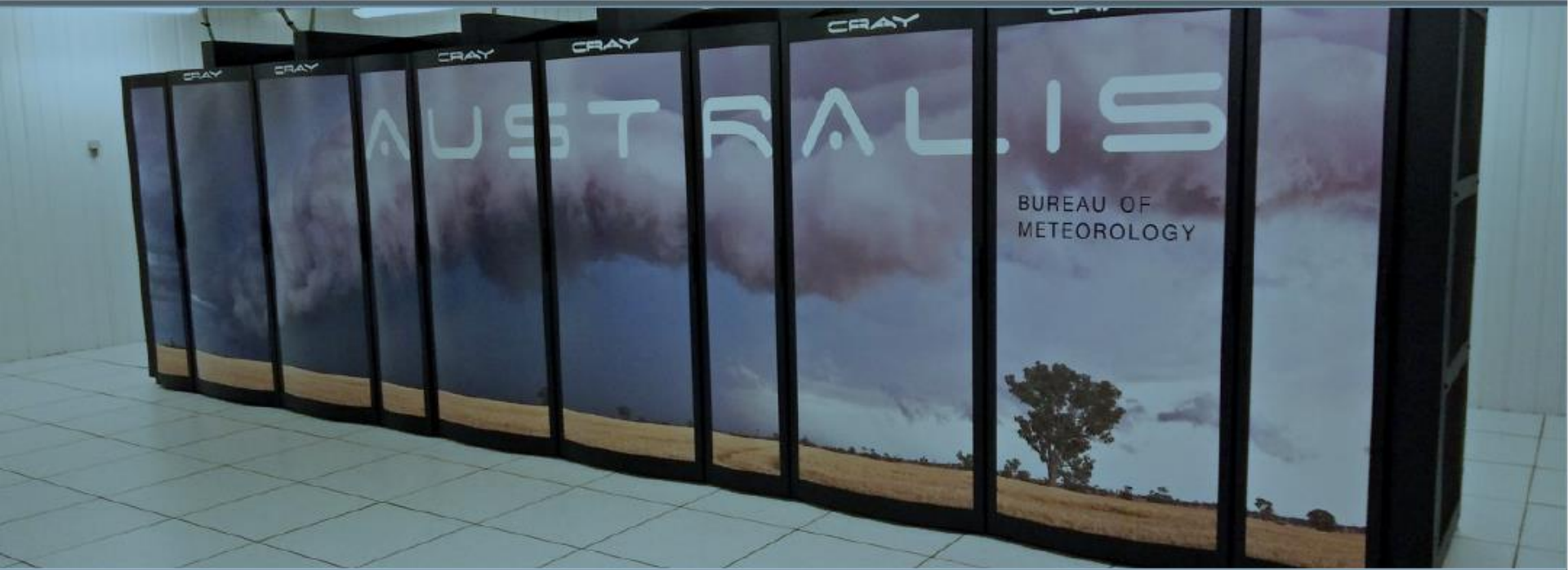
Figure 5. The Bureau of Meteorology's current Cray supercomputer. (Source: Tim Pugh, Bureau of Meteorology)
