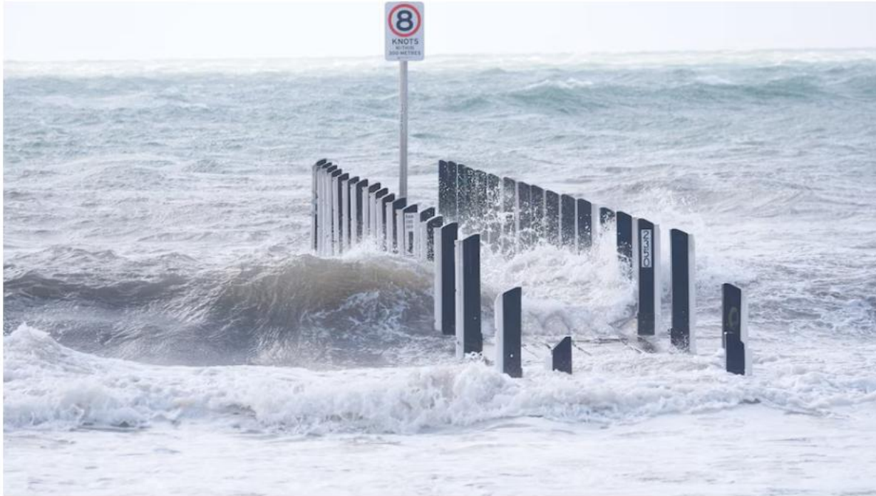
Quindalup boat ramp in WA's South West was left inundated as sea levels rose in the severe weather. (ABC News: Madigan Landry)
